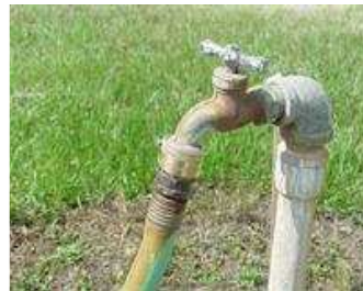
Figure 1. Vacuum breaker installed on hose spigot.
